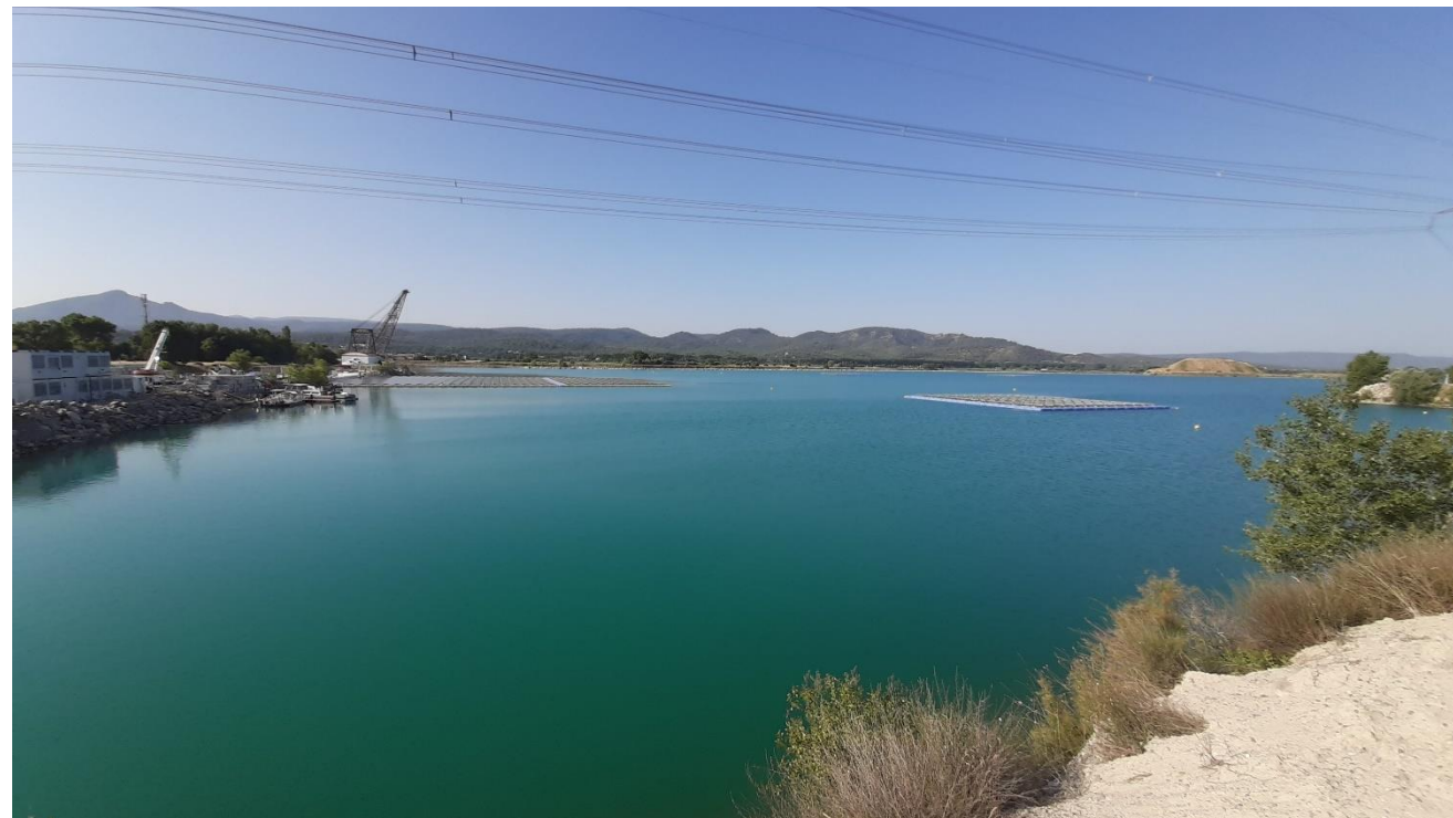
Figure 101 : Parc photovoltaïque flottant des Chapeliers (2/2)(BORALEX, 2021)
