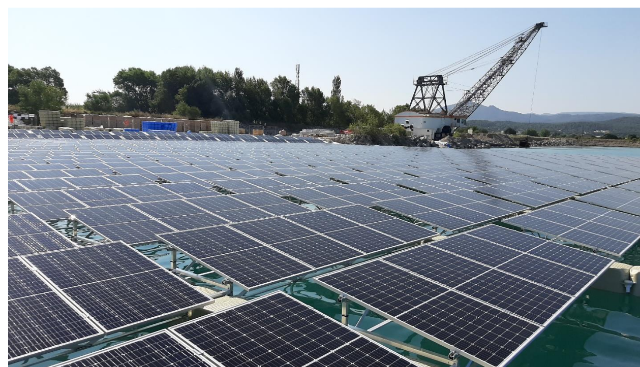
Figure 100 : Parc photovoltaïque flottant des Chapeliers (1/2) (BORALEX, 2021)
